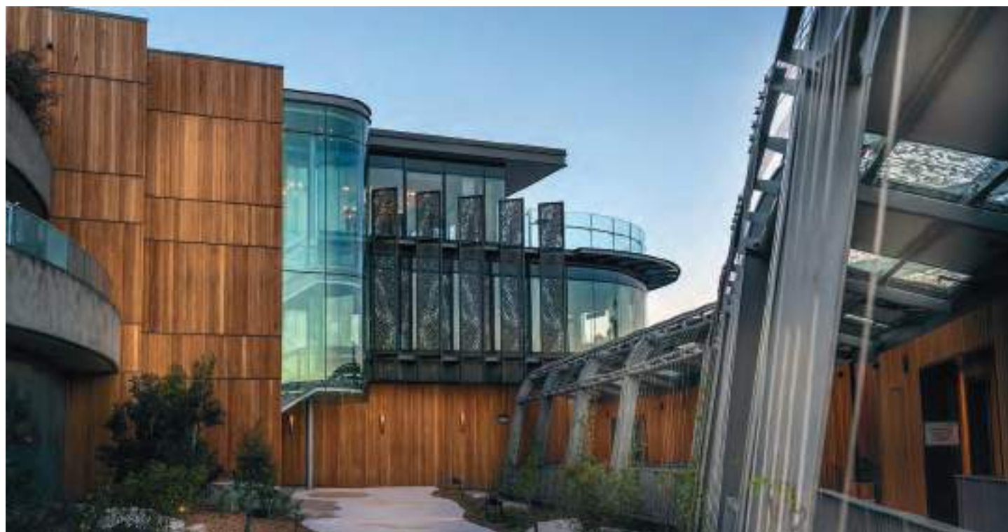
Above: A series of CLT pods ranging from two to four storeys deliver 62 guest rooms at Taronga Zoo’s recently completed Australian Habitat and Wildlife Retreat.
