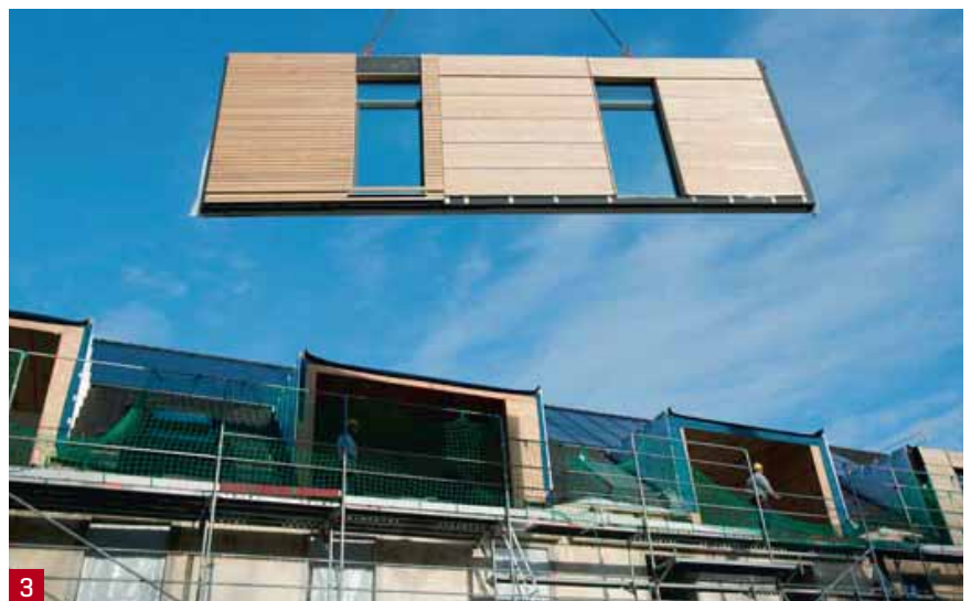
IMAGE 1: Australand Parkville five storey timber frame construction with floor cassettes. IMAGE 2: Pryda frame and truss fabricators now offering floor cassettes. IMAGE 3: Prefinished panel walls in Europe are common for multi-residential buildings.
